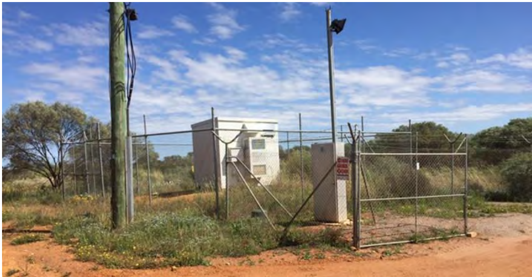
Figure 32. CSIRO's MRO fibre communications repeater hut at Mullewa
