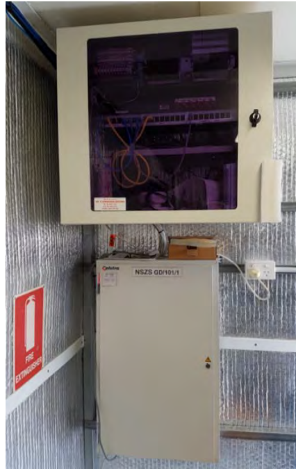
Figure 25. Telstra fibre communications access point
